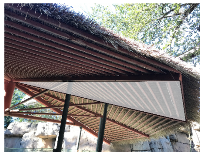
Photo SEQ Photo \* ARABIC \r 1 1 - Closeup of the penguin exhibit roof, highlighting one of the triangles that make up the roof. PC: Jonathan Fdauid
